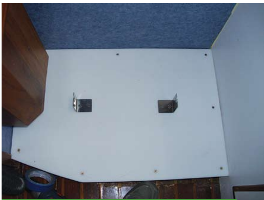
The old toilet platform with hose holes was sealed with epoxy. Next, it was edged and covered with 1/2" high density polyethylene (HDPE). Mounting clips for new head are in place
